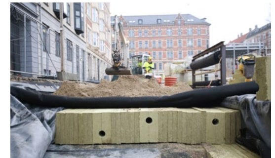
The photo underneath shows how Rockflow has been installed under the surface of the square. Unlike insulation, the stone wool in the Rockflow system is specially engineered to absorb and retain water. A system of pipes and gullies bring the storm water to the stone wool buffer where it is absorbed quickly and released slowly, either to the sewer or surrounding soil.
